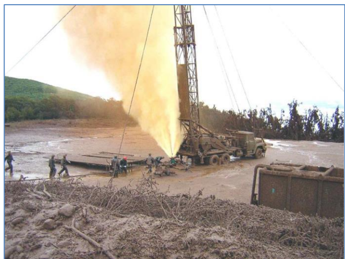
Figure 3-1 Inland well blowout while being decommissioned. Source: www.archive.epa.gov
