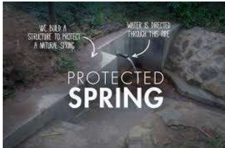
Figure 33: Example of a protected spring (thewaterproject.org)
