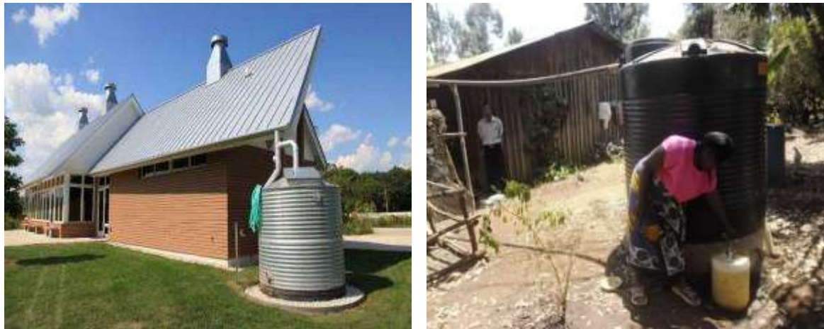
Figure 34: Examples of rainwater harvesting facilities
