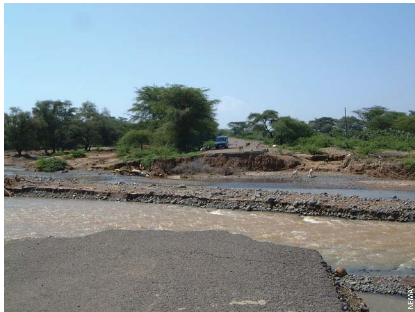
A section of a road in Baringo damaged by floods.
