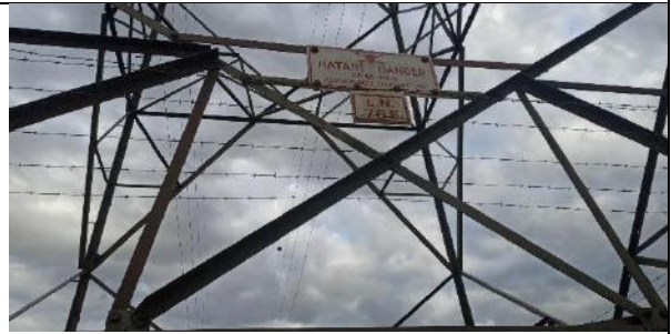
Tower 764 near power line exit area from the Park
