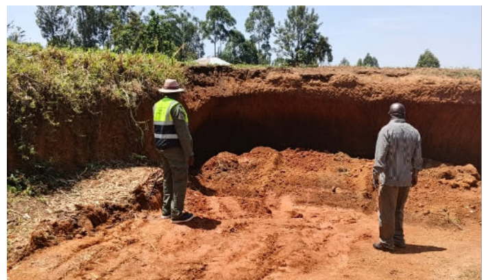
NEMA Board Member, Maclean Sitati (L) accompanied by a local inspecting the abandoned and non-rehabilitated sections of the pit in Webuye.
