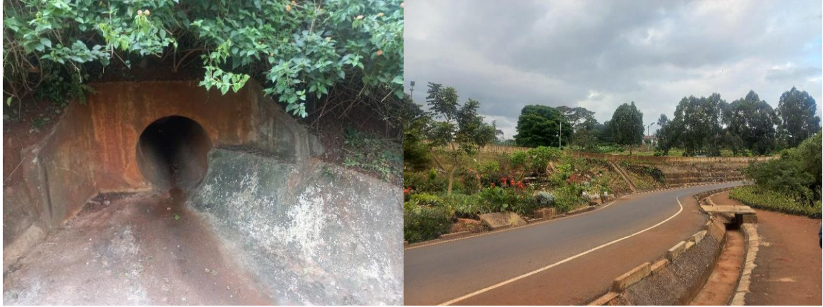
Well-built storm drains and a view of the Red Hill Link Road
