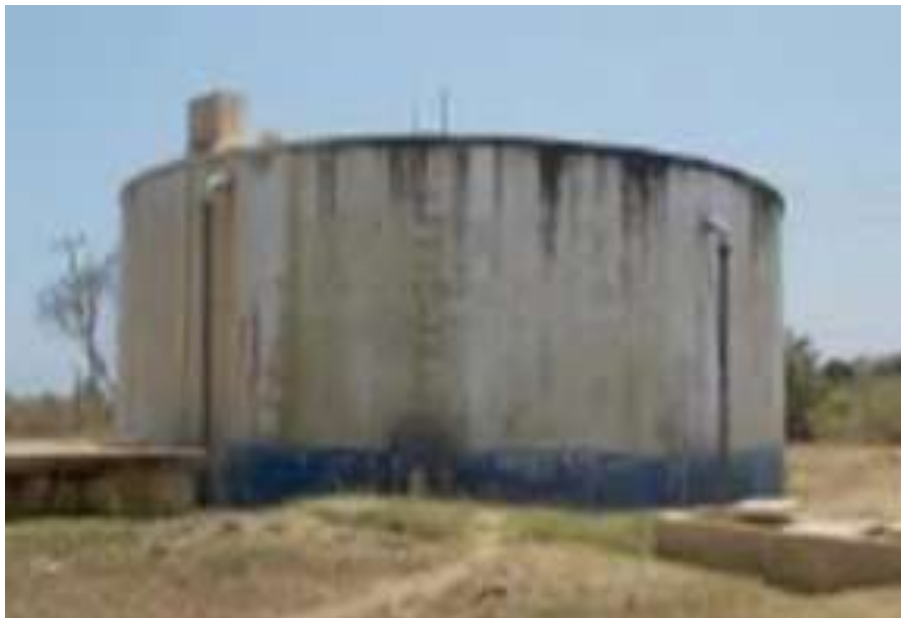
Figure 14: Kaya bombo reservoirs which is 1250m 3 tank and 2Nr which is 1,440m 3 tank
