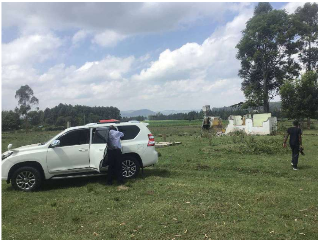
Plate 2: Site access during the assessment, showing the derelict remains of the former public works buildings on the parcel.
