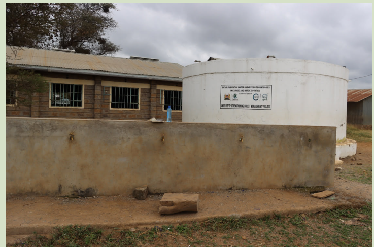
10,000 Litres masonry Water Tank at Ol dunguro Primary School in Kajiado County.
