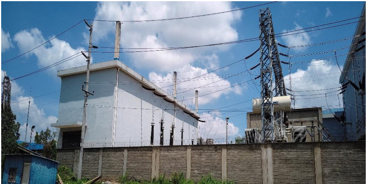
Plate 19: Kenya Power 220KV Substation (Source: Fieldwork by Orwe Elly)
