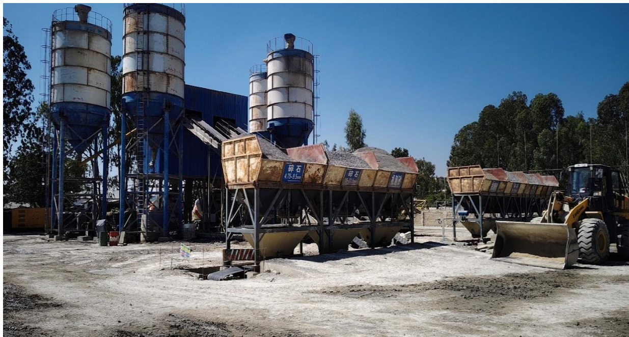
Plate 11: Existing Concrete Batching Plant (Source: Fieldwork by Orwe Elly)
