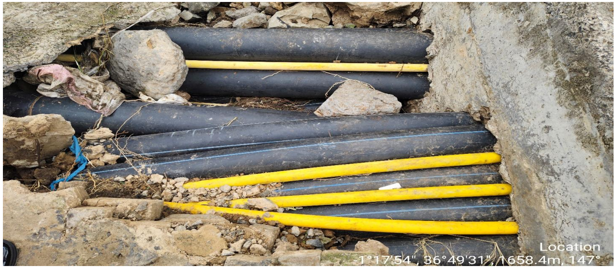
Plate 21: Exposed Section of High-voltage KPLC Underground Transmission Line (Source: Fieldwork by Orwe Elly)
