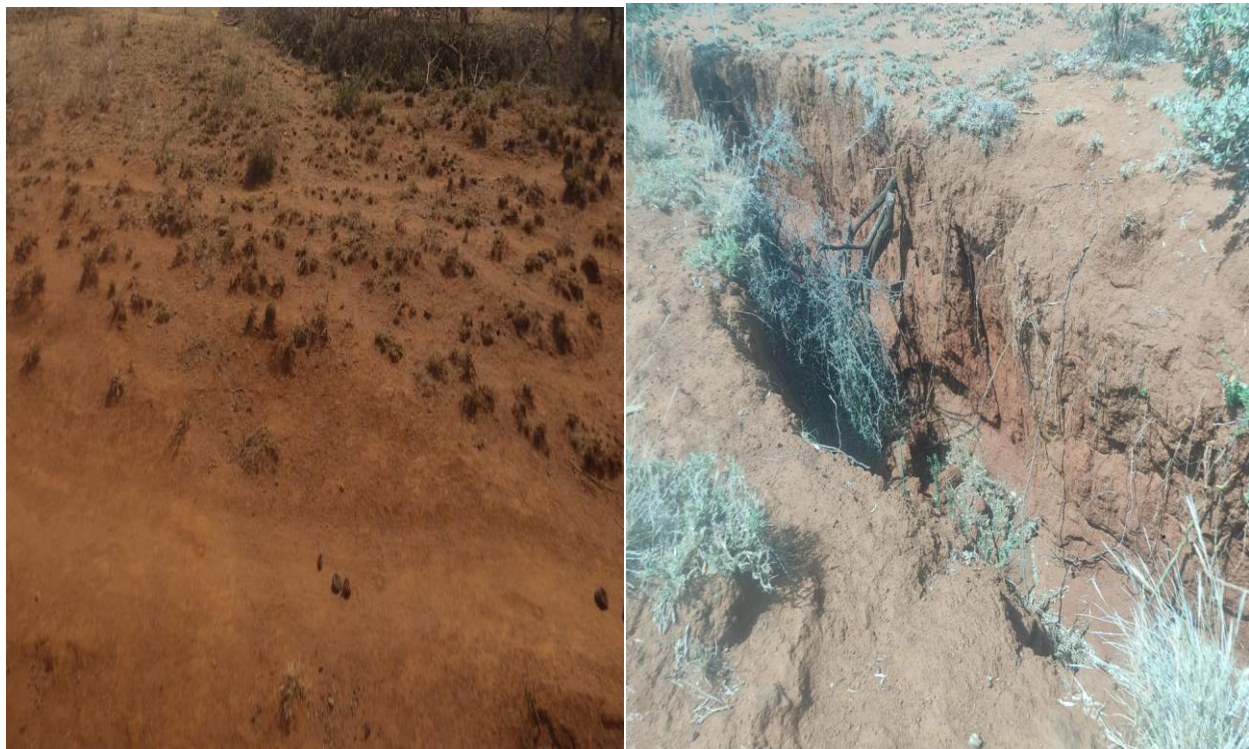
Photo 8: The soil type in the area that is susceptible to wind and gully erosion
